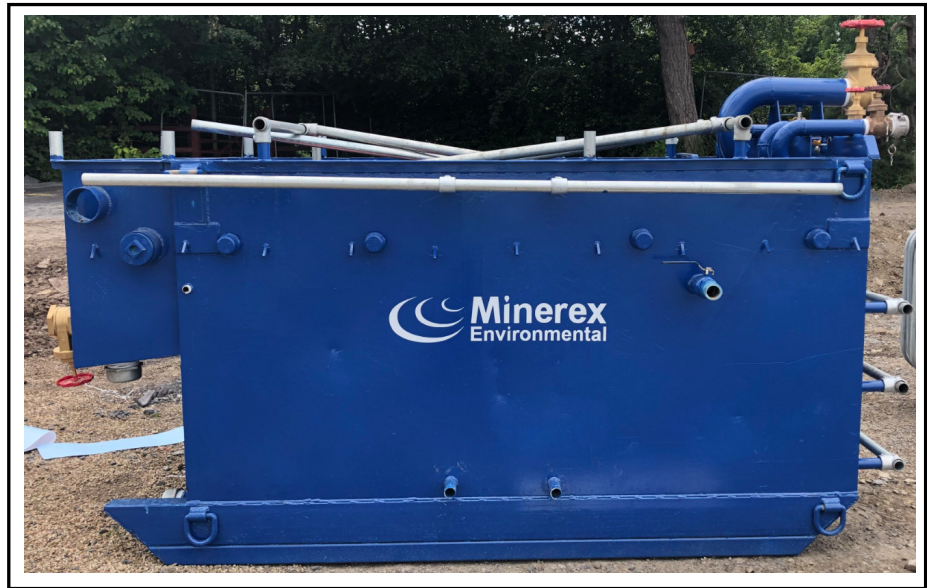
Example of an oil-water separator Minerex Environmental Limited, an RSK Group company
